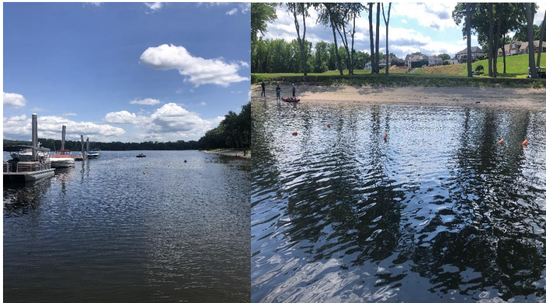
Figures 3 and 4. River Highlands site in Cromwell, CT during benthic barrier installation, 2022.
